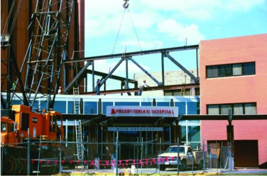
Framing for a new three-story pedestrian bridge over the existing lobby is erected.
